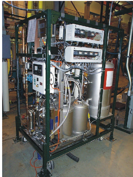
Figure 5. Photograph of the prototype water cooling and temperature control skid.
